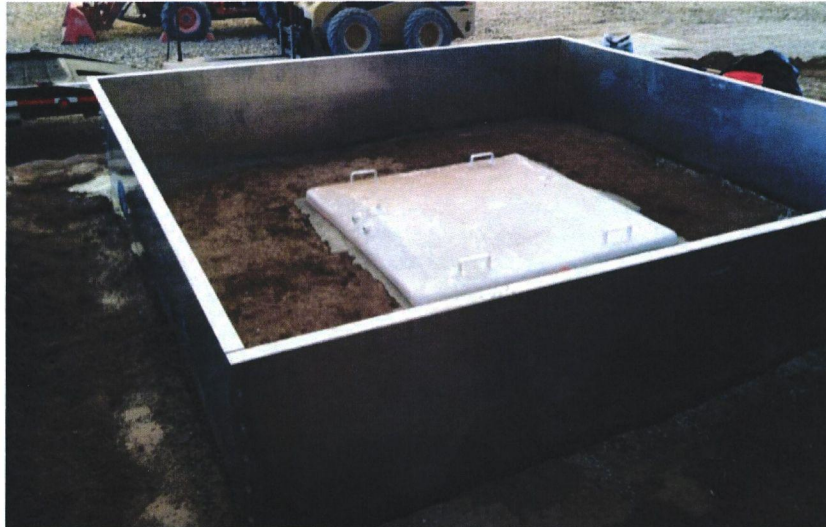
Figure 1 – SDRI test equipment installation prior to being filled with water
